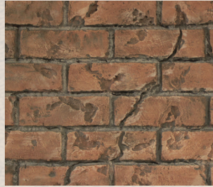
Fire Cracked Brick
