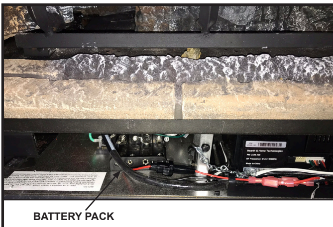
Figure 3.8 Battery Pack Installed
